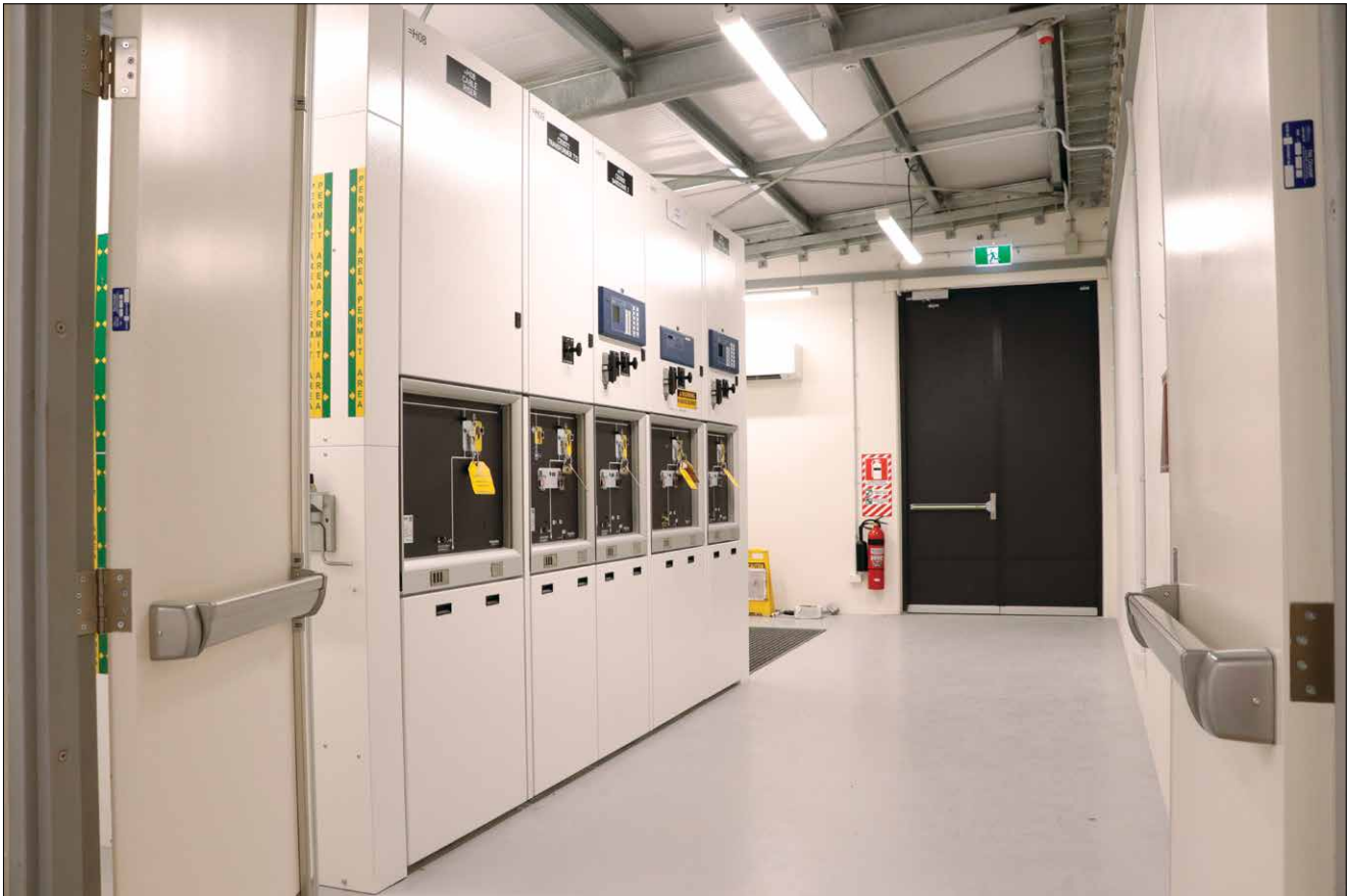
Figure 113: 33kV and switchgear panel circuit breakers
