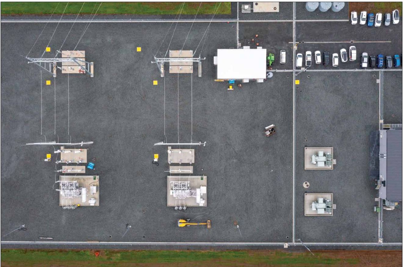
Figure 111: Power transformers at the Forrest Road substation
